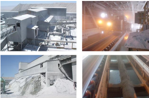
Figure 15: Closed Copper Ore Stockpile with Tripper Car Feeding
